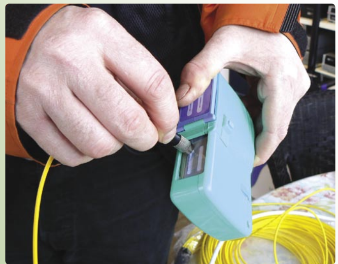
A word of caution to all installers: Never simply plug in optical cables – the connections of the cables need to be perfectly clean before they are put together. Various methods can be used to achieve this; the most practical is using the device shown here: the connector of a fibre optical cable is inserted and a lever is then operated to clean the connector with an extremely fine-grain abrasive paper that is only used once. This is the only way to guarantee a plugged connection is established without any signal attenuation.
