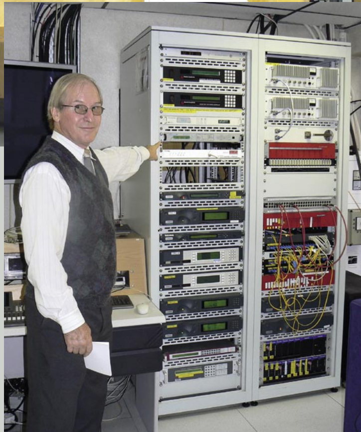
▲ Clive Grove is Telemedia's Project Engineer. Here he shows us the cabinet with all the encoders. Clive comes from England and installs satellite antennas in many African countries. He is also a TELE-satellite writer!
