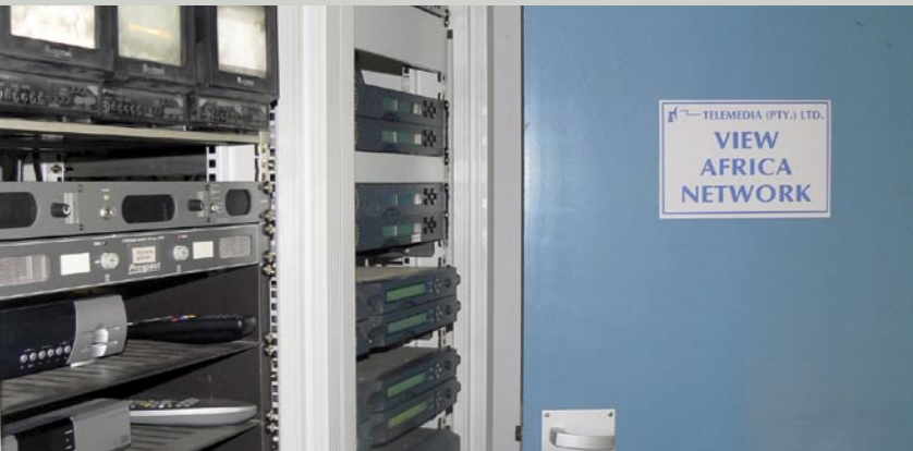
▲ Here is the heart of the View Africa channel package: reception monitors and receivers can be found in the cabinet to the left while the right-side cabinet houses the various encoding slots for all the different channels. The feeds for many of the channels originate from the studios that are only a few steps away.
